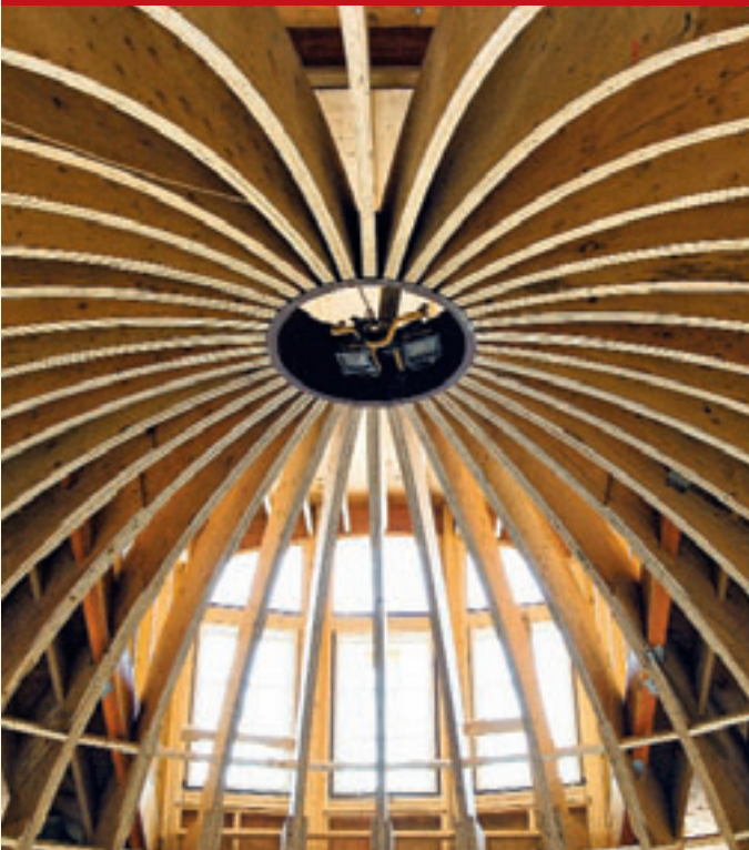
Pyramid Builders portfolio includes a waterfront home with a pool house (top) and a barrel-vault ceiling with an elliptical window (above, during construction).
